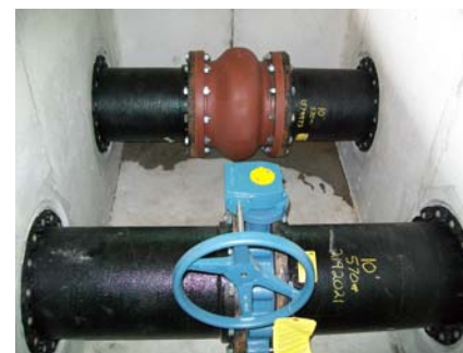
Nelsey Road Booster Station Project. Completed in Operational Year 2010. The Station elevated water pressure for customers within its service area by an average of 20 PSI.
