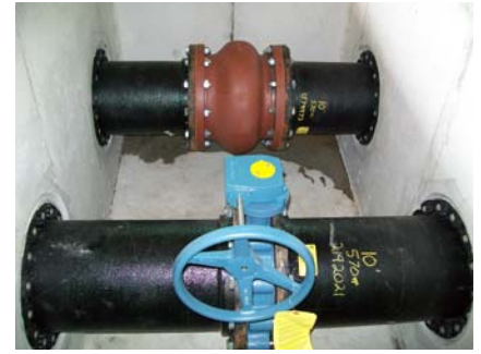
Nelsey Road Booster Station Project. Completed in Operational Year 2010. The Station elevated water pressure for customers within its service area by an average of 20 PSI.
