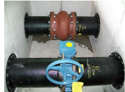
Nelsy Road Booster Station Project. Completed in Operational Year 2010. The Station elevated water pressure for customers within its service area by an average of 20 PSI.
