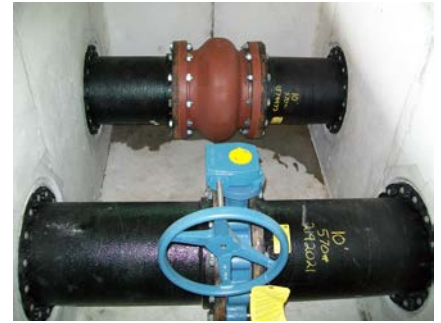
Nelsey Road Booster Station Project. Completed in Operational Year 2010. The Station elevated water pressure for customers within its service area by an average of 20 PSI.
